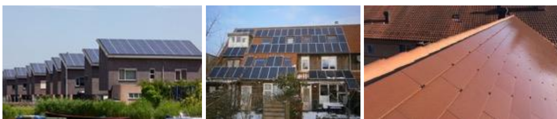
Figures 14, 15, 16. Residential rooftop PV arrays
