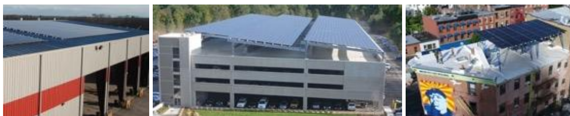
Figures 8, 9, 10. A selection of large continuous rooftop PV arrays
