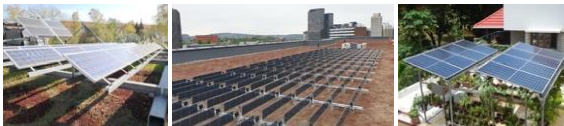
Figures 11, 12, 13. PV + vegetation on roofs
