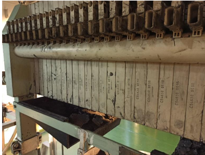
Figure 4. View of a filter press from a hybrid EGCS installed on board of a ship. Source: The Authors.
