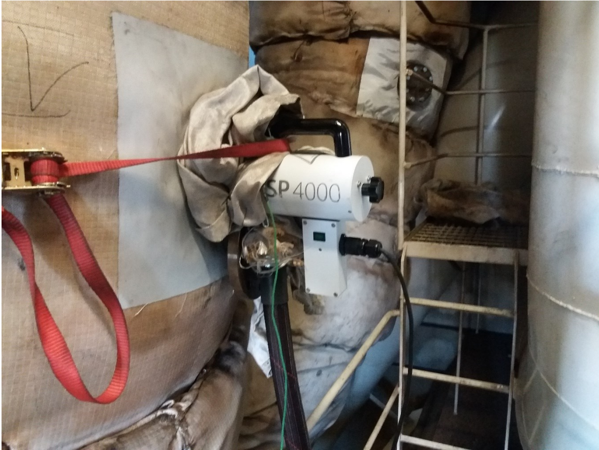
Fig. 2 Measuring probe installed in the stack (another measuring flange is found in the background)
