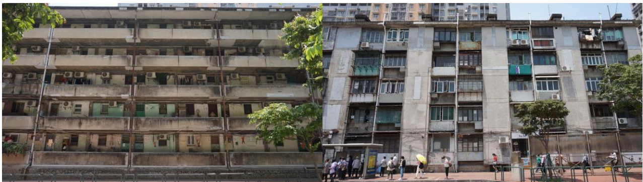
Fig. 10 "Affordable Housing of Ilha Verde Area" Typology. Personal Picture, N. A. Galliano (2023). Fig. 11 "Affordable Housing of Ilha Verde Area" Typology. Personal Picture, N. A. Galliano (2023).
